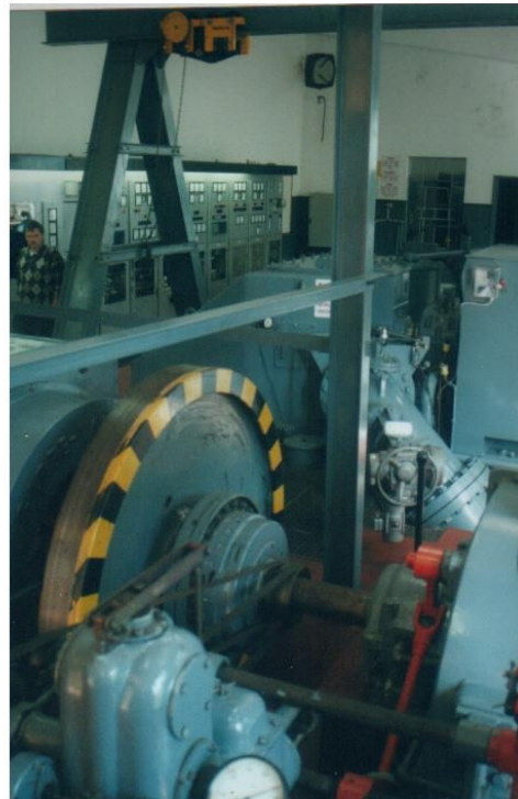
Interior of 2MW Lydenburg plant
