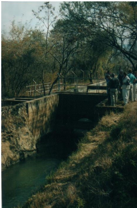
Feeding canal headrace
